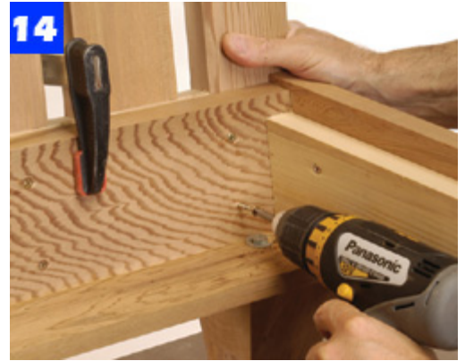
14 Temporarily clamp the chair back to the base and fasten the parts with galvanized deck screws.
